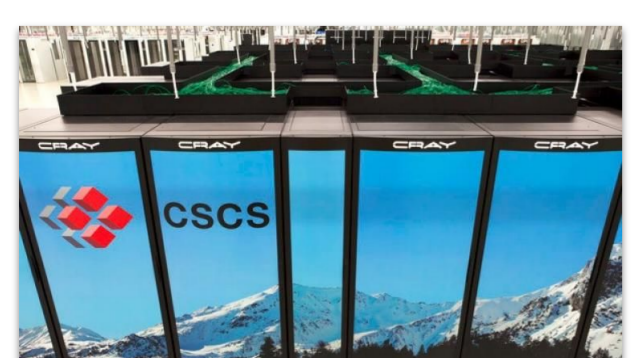
Piz Daint @ Swiss National Supercomputing Centre (Switzerland)
